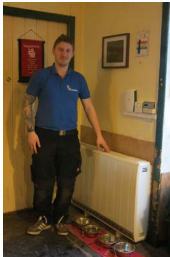
RS Merriman's electrician Kevin with newly installed Quantum heater at Quoys, Rousay
